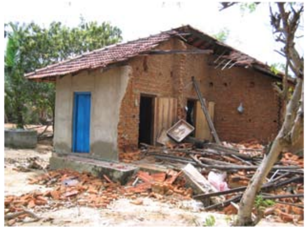
Figure 7: Partially collapsed brickwork structures due to tsunami tidal waves in Sri Lanka
