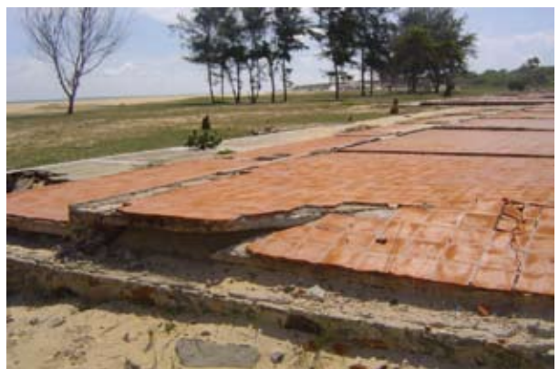
Figure 9: Failure of a masonry low rise building in Yala-Safari Beach Hotel, Yala, due to tsunami waves
