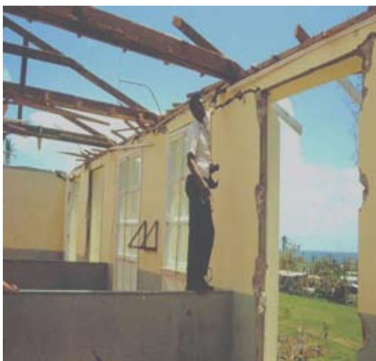
Figure 13: Single storey building; asbestos roof has blown away due to a cyclone
