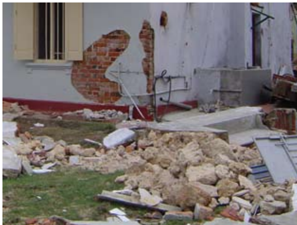
Figure 12: A house close to the shoreline, its short and stiffer edge facing towards the sea
