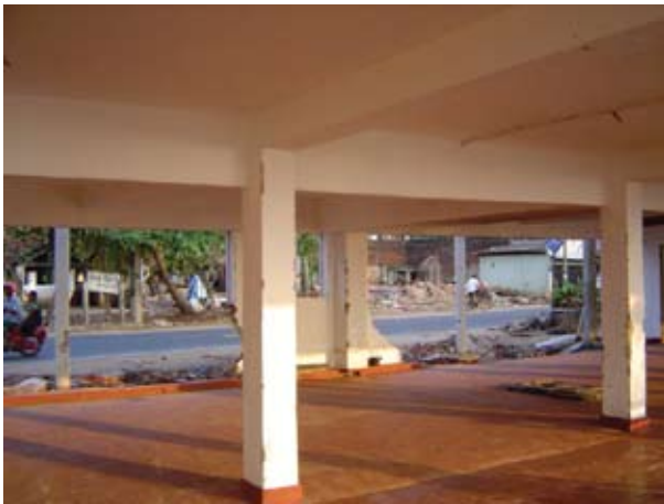
Figure 8: A structure of a building survived with minimum damage. Only the infill masonry panels have collapsed from tsunami waves
