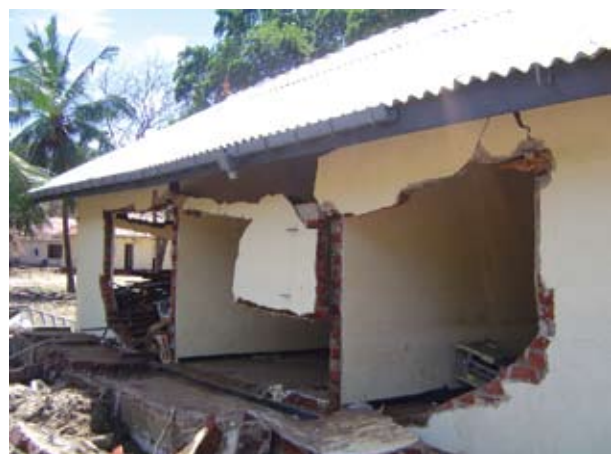
Figure 11: A house close to the shoreline, its long weaker side facing the sea coast
