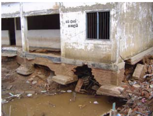
Figure 10: Under-scouring of foundation at a corner of a school building from tsunami waves
