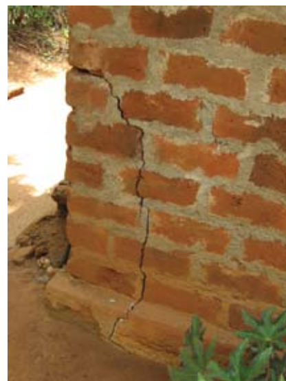
Figure 17: A masonry house subjected to earthquake induced ground motion- Beralihela, Tissamaharama
